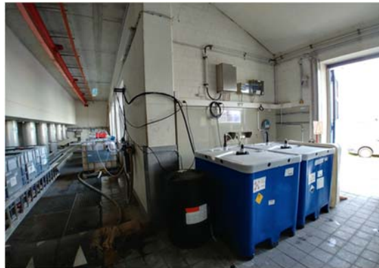
Chlorine dioxide pilot plant
